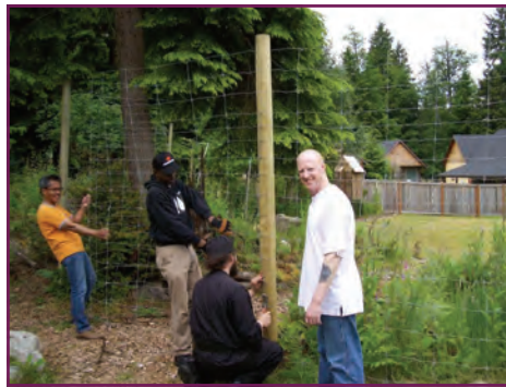
Jonathan, Johnny, Fr. Moses, and Larry installing a fence to keep the deer out
